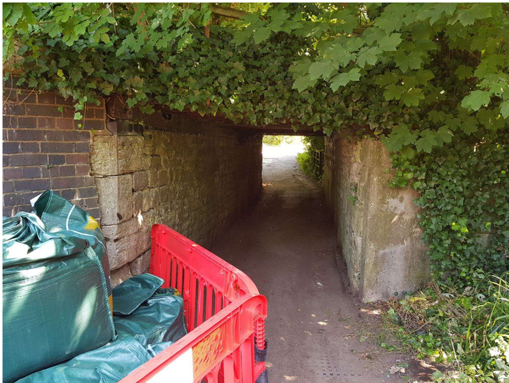
The Picture above shows the implementation of emergency gravel bags to hold up the deteriorating bridge wall.
